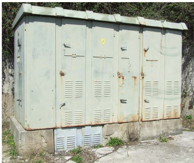
BTS 10/0.4 kV Markovići
