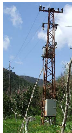
STS 10/0.4 kV Mažići
