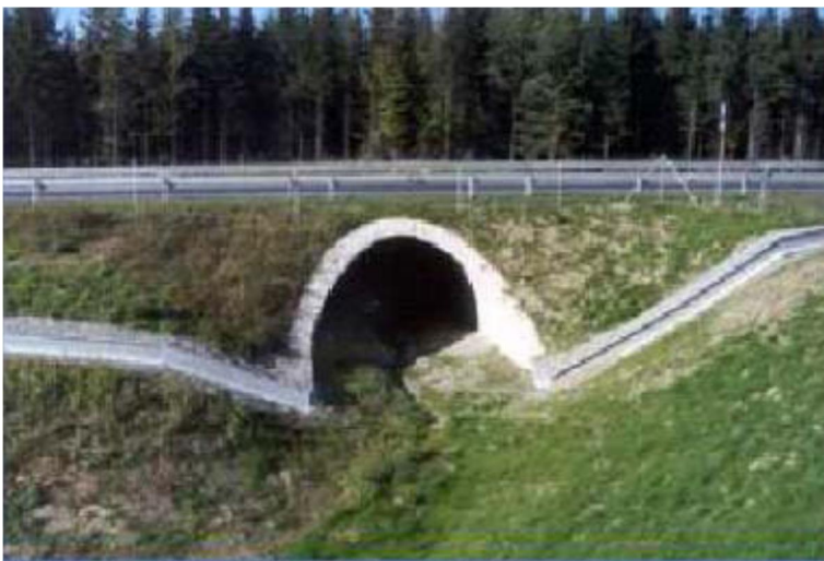
Arch culvert with fence for large mammals and lipped wall for amphibians (FHWA/US DOT, 2002)
